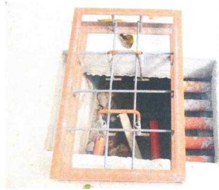
Debris inside the canals
