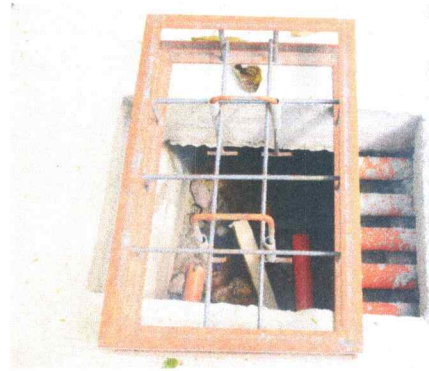
Debris inside the canals
