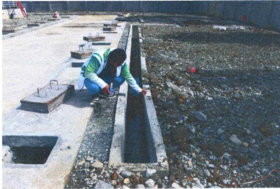
No brace meters and have cracks in line canal
