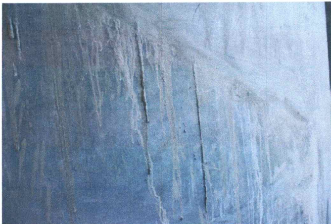
Hardened cement residues on walls
