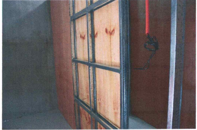
Infrequent placement of steel frame division
