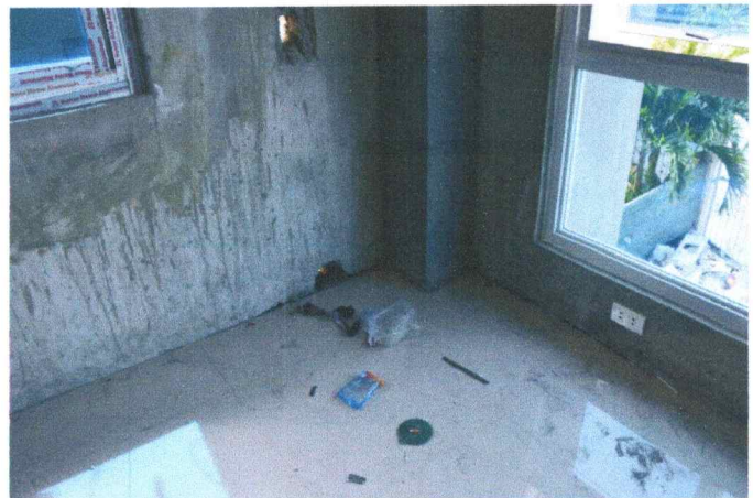
Incomplete tiling specially in the corners
