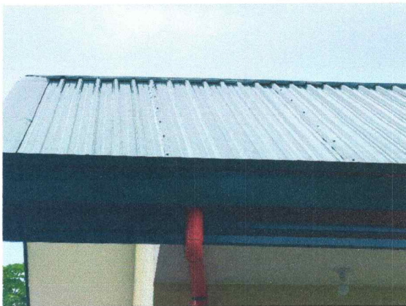
Insufficient texscrew for the roofing installation
