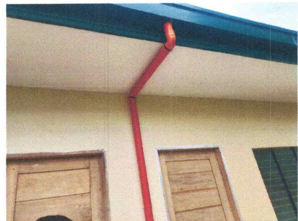
Water leak in the gutter
