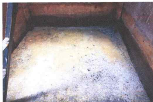
Loose concrete mixed
