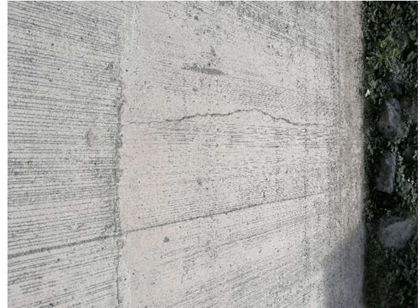
PCCP blocks with transverse cracking within 1.5 meters from weakened plane joints
