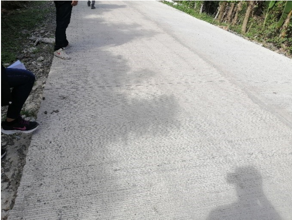
PCCP blocks with transverse cracking within the middle block
