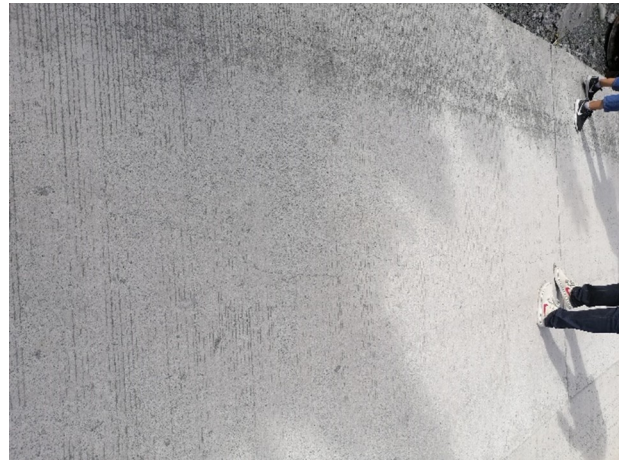
PCCP blocks with longitudinal crackings
