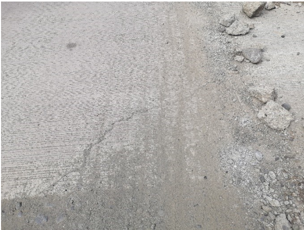
PCCP blocks with transverse cracking acting as weakened plane joints
