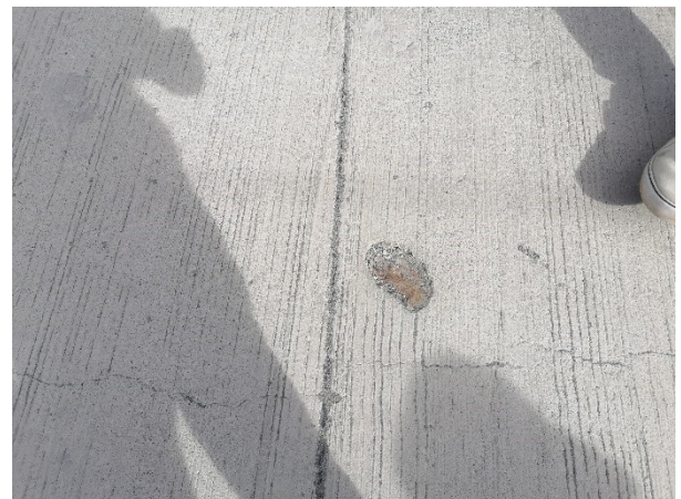
PCCP blocks with pockmarks
