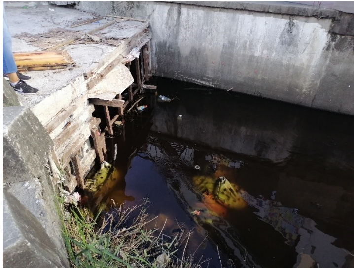
Unremoved forms and scaffolding works
