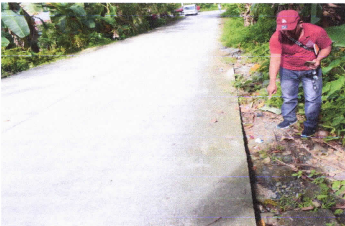
Weak Road Shoulder
