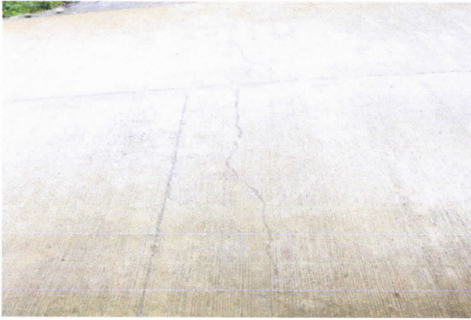
PCCP blocks with transverse cracking within the middle block
