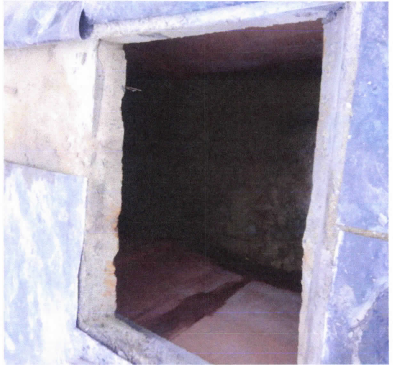
Vault had water and some debris
