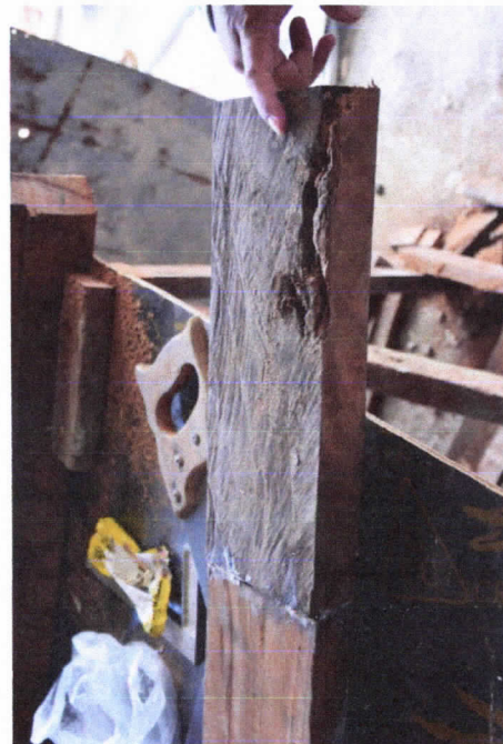
Door Jamb with Termites
