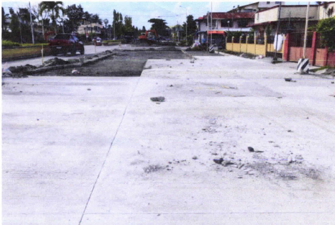
Water Ponding in some portions
