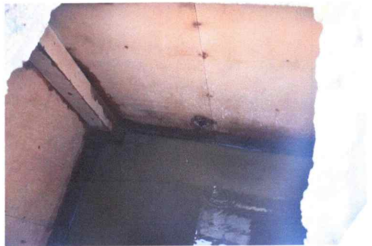
The septic vault still had water and damaged corkboard
