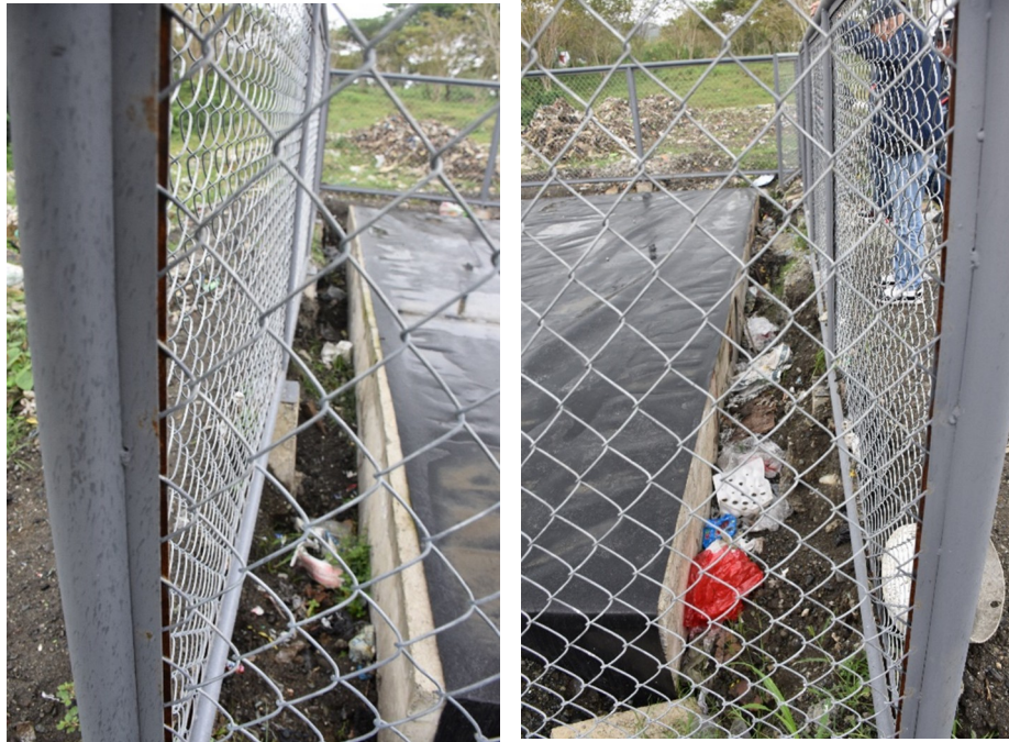
Incomplete installation of liner (2 sides)
