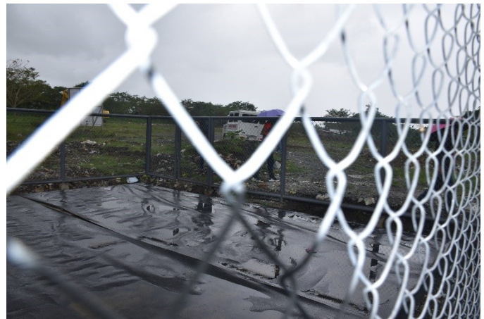
Inappropriate installation of manhole cover
