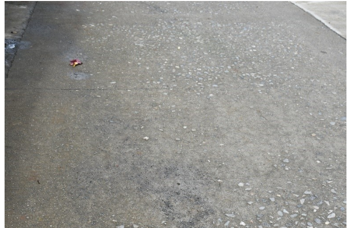
PCCP blocks with major scaling
