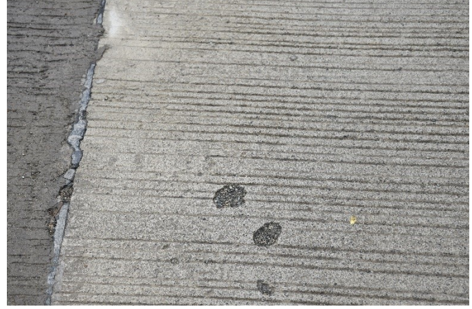
PCCP blocks with pockmarks
