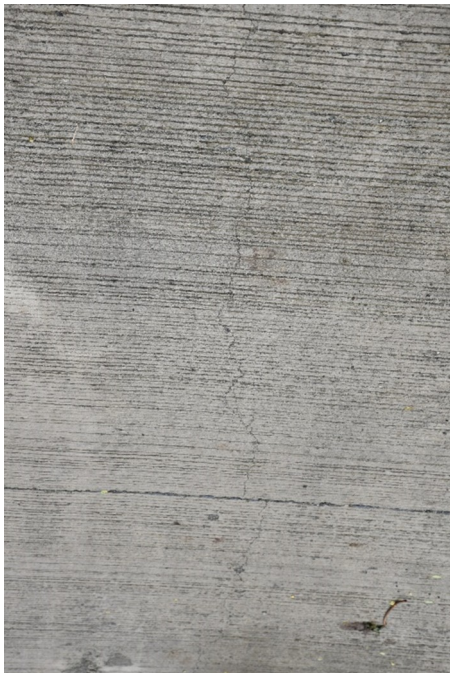
PCCP blocks with longitudinal crackings
