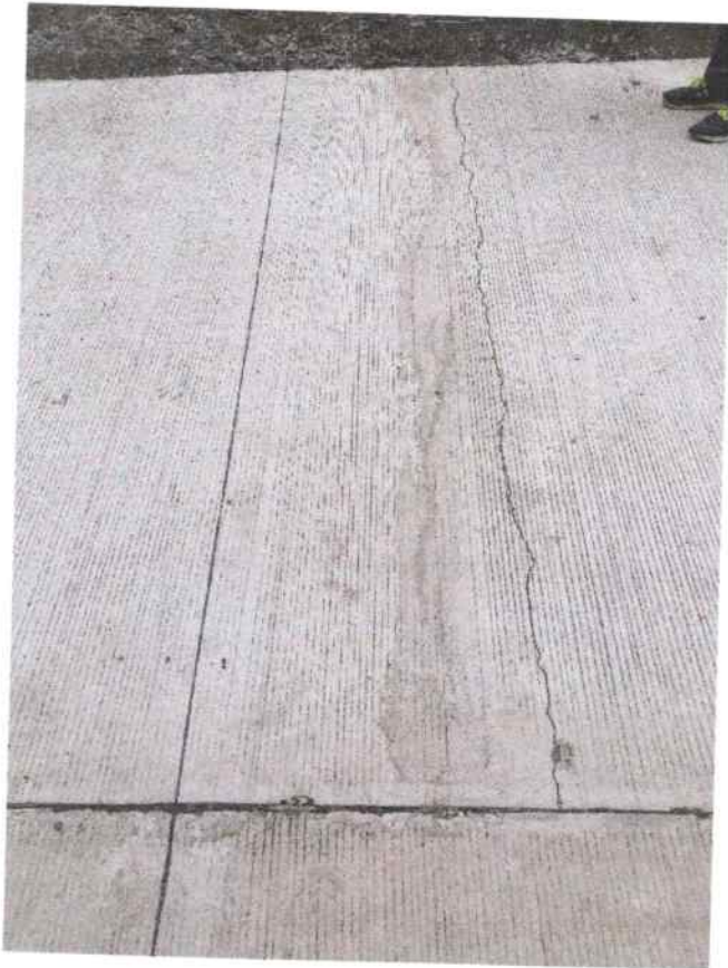
PCCP block with transverse cracking within 1.5 meters from weakened plane joints
