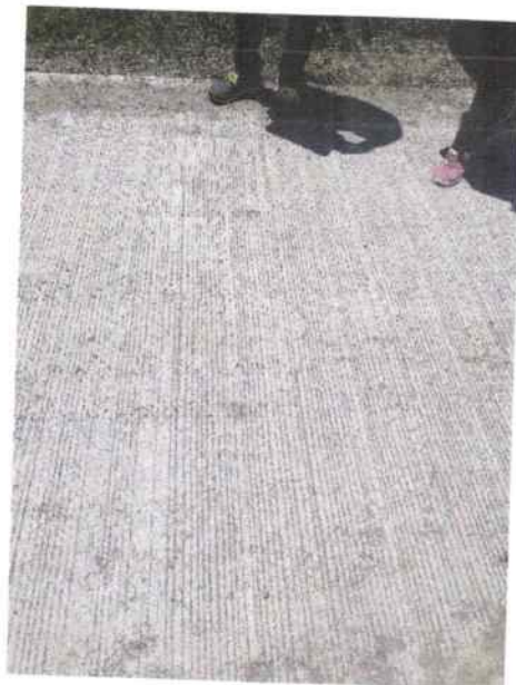
PCCP blocks with transverse cracking within the middle block
