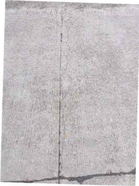
PCCP blocks with transverse cracking acting as weakened plane joints
