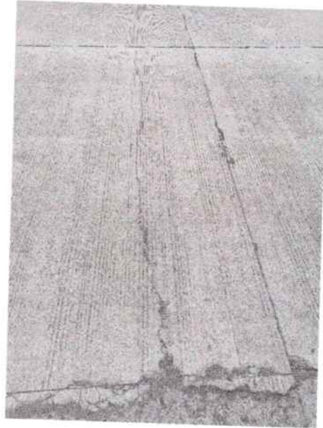
PCCP block with transverse cracking within 1.5 meters from
