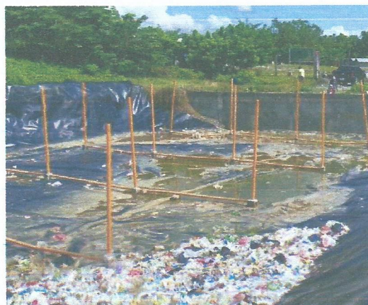
Detached part of liner
