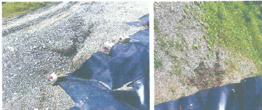
Presence of waterway causing water intrusion to the project
