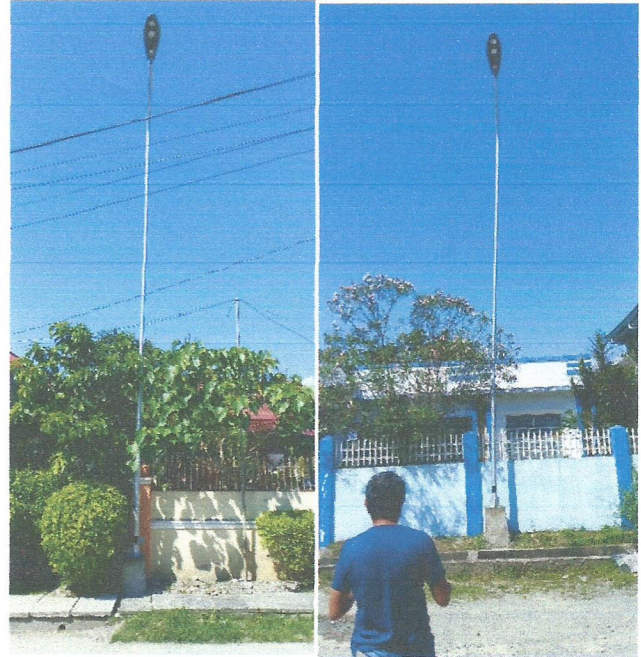
Some posts are slanted
