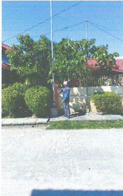
Location of streetlights at Remedios Street do not match to the approved Layout Plan
