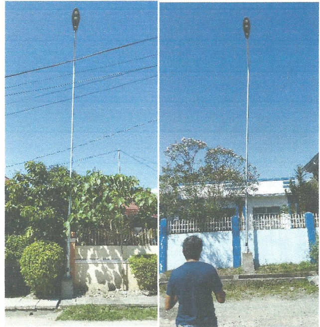
Some posts are slanted
